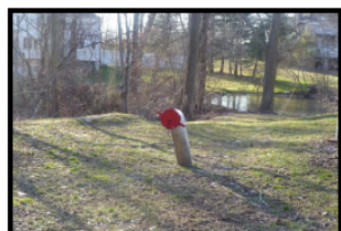
Dry hydrant on Braeburn Drive
