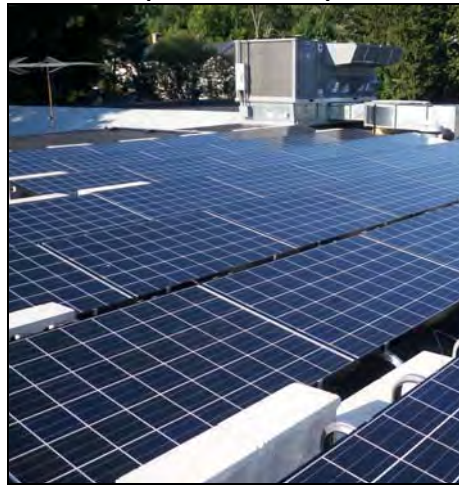
Rooftop Solar Installation (Karl Chevrolet)
