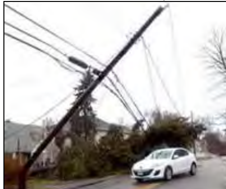
Electrical Service Interruption
