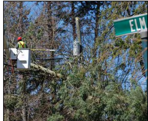
Electrical Service Interruption
